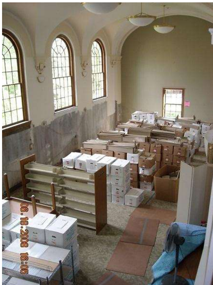
The renovation project was all encompassing, but progressed quickly. The Main Reading Room in June, 2008.
